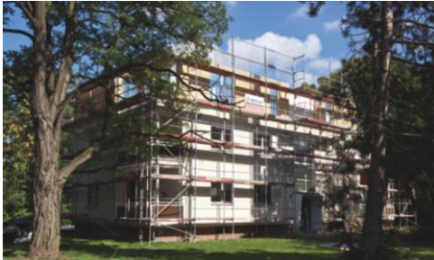
In the Berlin borough of Tegel, wood-based materials from KRONO were used to add a storey and create healthy, energy-efficient living space.
